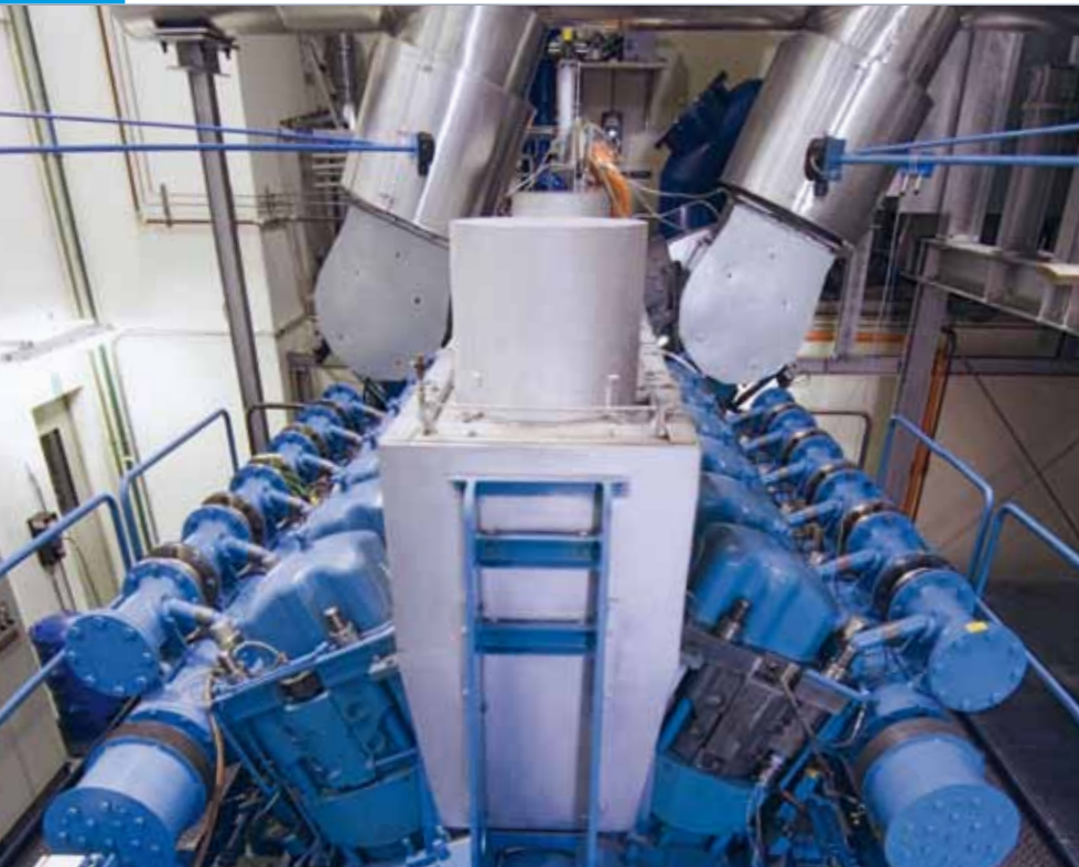
MAN Diesel & Turbo operates its own industrial co-gen plant at its Augsburg works, where diesel and gas engines provide electrical power for the foundry furnaces, process heat and district heating.
